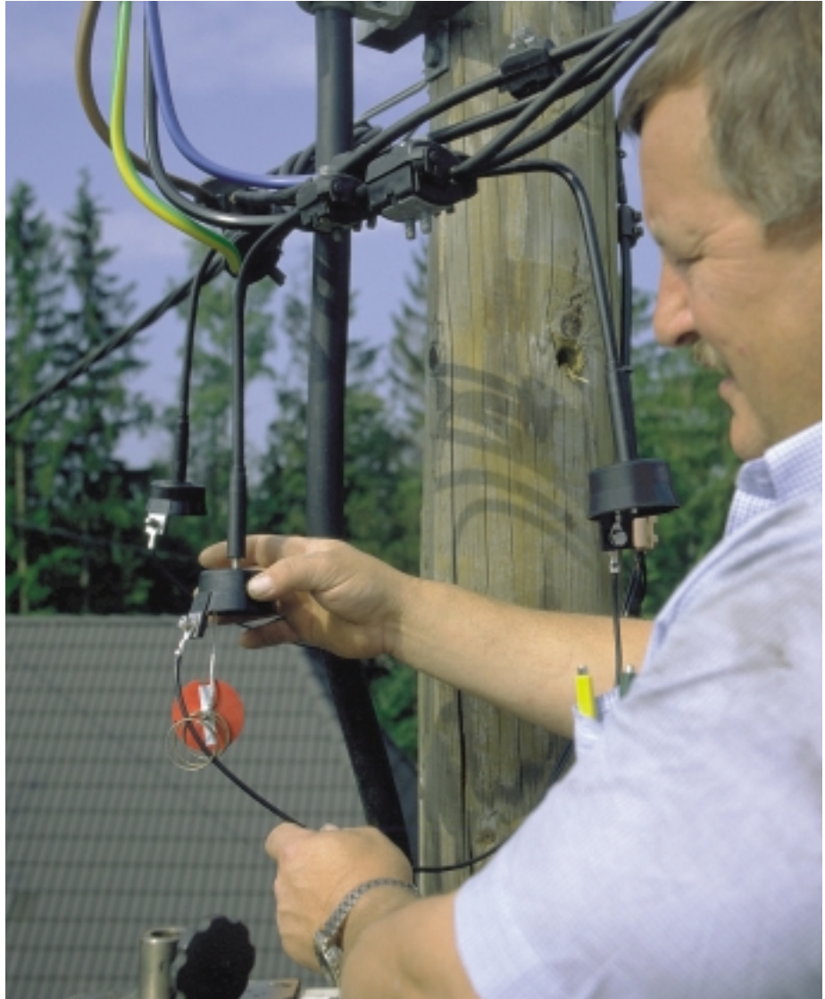
Transition: insulated overhead lines to cables
