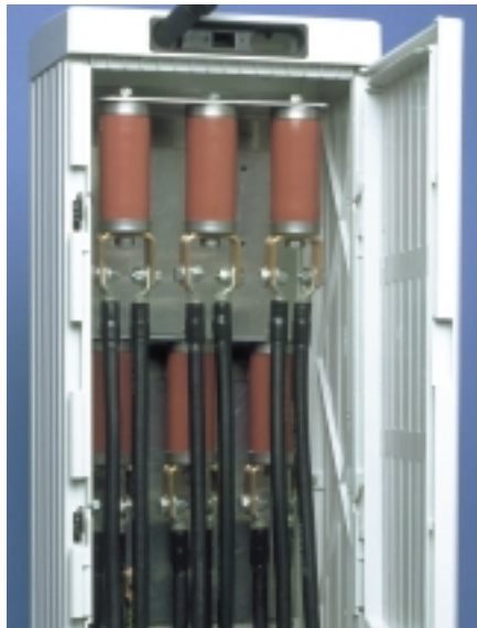
CPA arresters installed in a cubicle to protect HV cable sheath cross bonds
