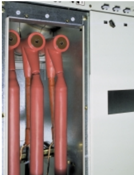
Gas-insulated switchgear with RDA arrester
