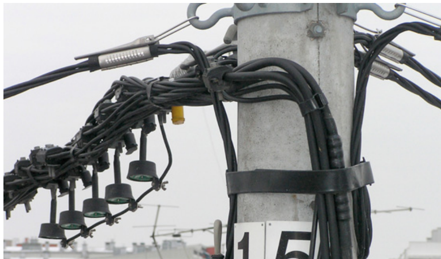
Transition: insulated overhead lines to cables
