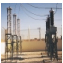
HV surge arresters
